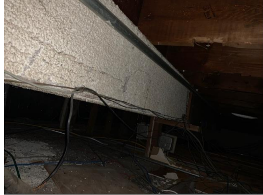
Photo of HA number 26, Sample No. 0206-26-84, 85, 86 | ACM White Fireproofing, within Crest Station 18 Roof
