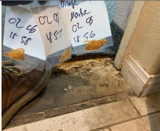
Photo of HA number 18, Sample No. 0206-18-56, 0206-18-57 & 0206-18-58 | Non-ACM Orange Carpet Mastic, within Open Room
